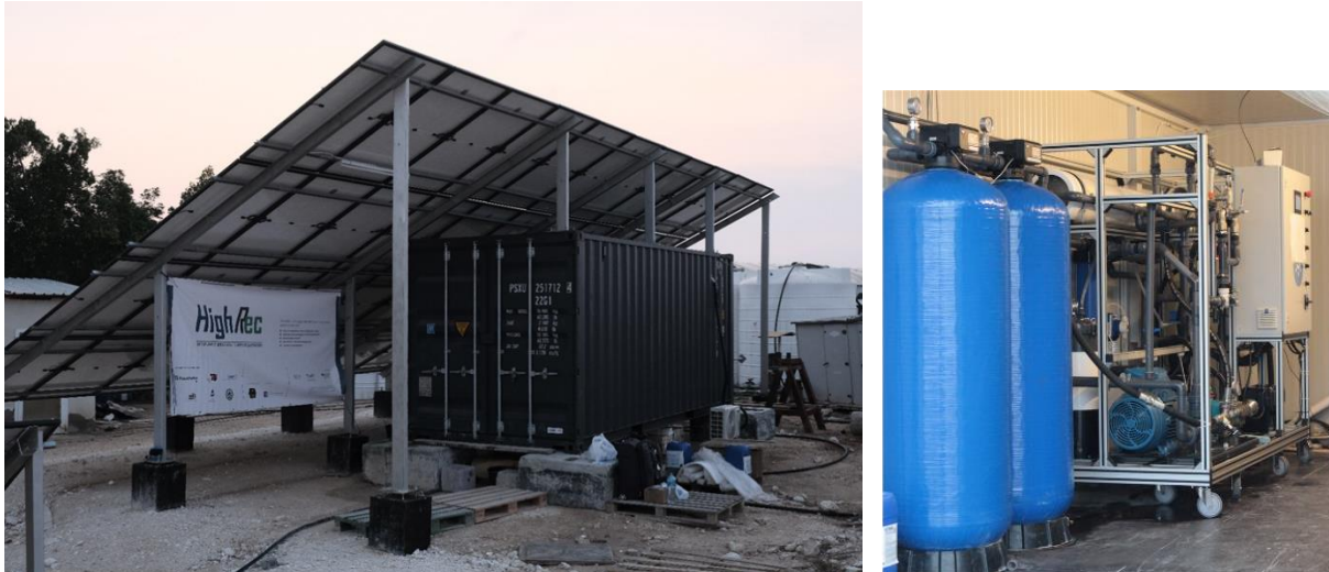
Figure 1: Container with CLRO under a shadowing rooftop of 44 photovoltaic panels at the horticulture farm Agrico, Qatar.
