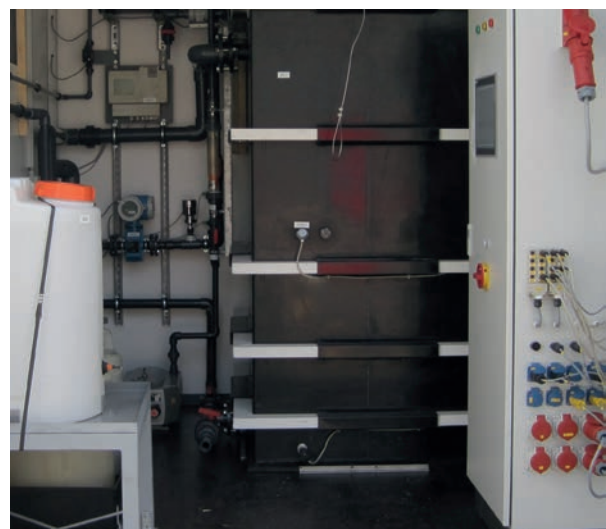
Within the joint project PU 2 R, domestic wastewater is treated in a mobile membrane bioreactor (MBR)
