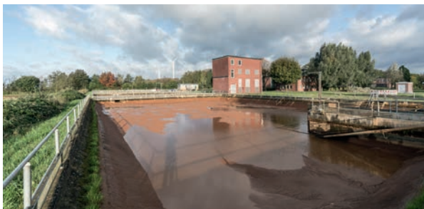
Settling basin for backwash water. With the water drained away, the sludge that has settled on the basin floor is clearly visible.
