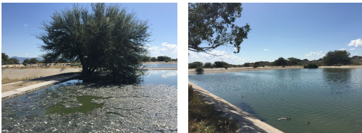
Figure 5: View to the anaerobic pond (left) with layer of floating material and plastic bottles and the facultative pond (right), (Foto FiW)
